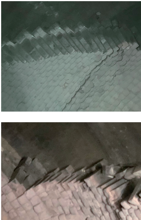
Fig. 8 Residual of more than 300 mm.
